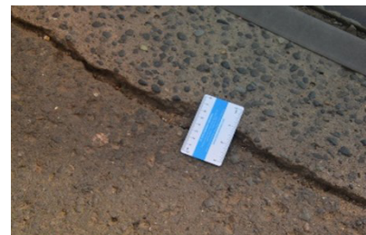
Fig 1b. Surface crack at the end joint
