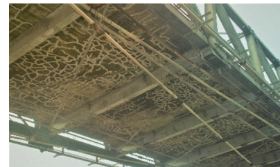
Figure 1a. Crack damage pattern at the bottom slab
